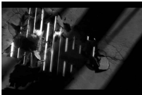
Figure 5.7. Screen shot: Hole in ceiling in Precious .
