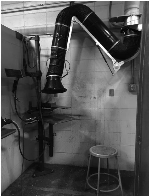
Figure I.13. Ventilation in a booth at NTC.
